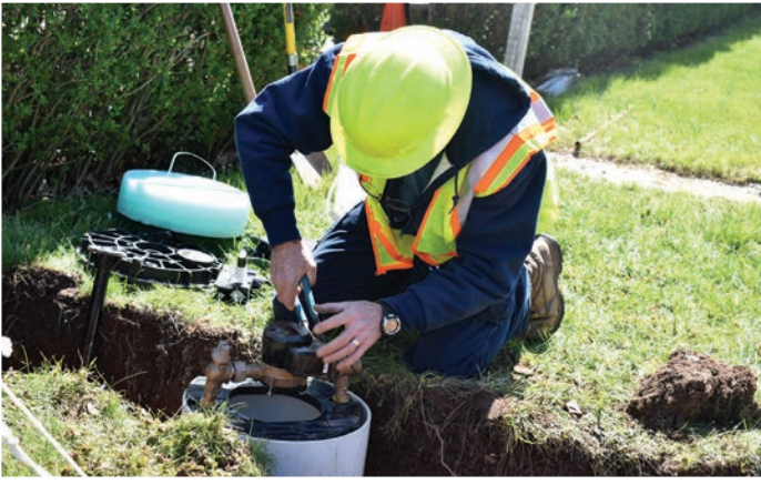
A North Penn Water Authority Field Service Representative installs a new meter in a meter pit, outside of a customer's home
