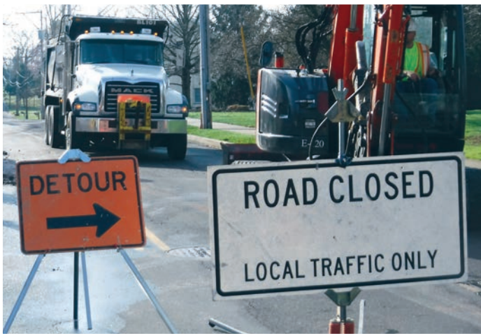
Road closure due to main extension on Township Line Road in Skippack
