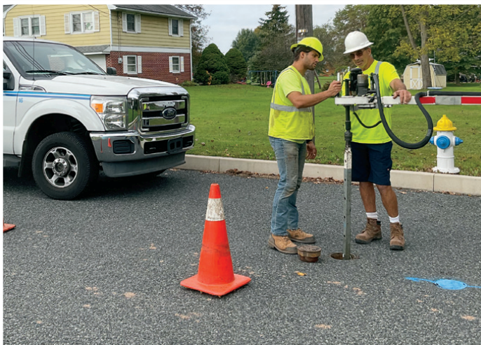
A veteran employee shows a newer employee how to exercise water valves.
